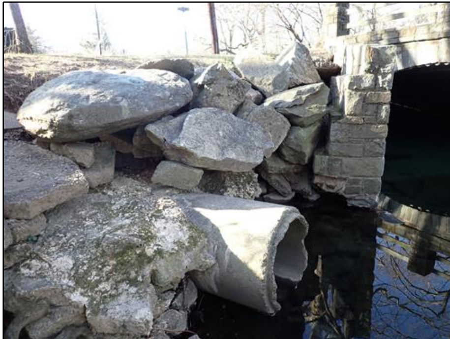
20. Southeast Embankment - Voids in Riprap Behind Southeast Wingwall
