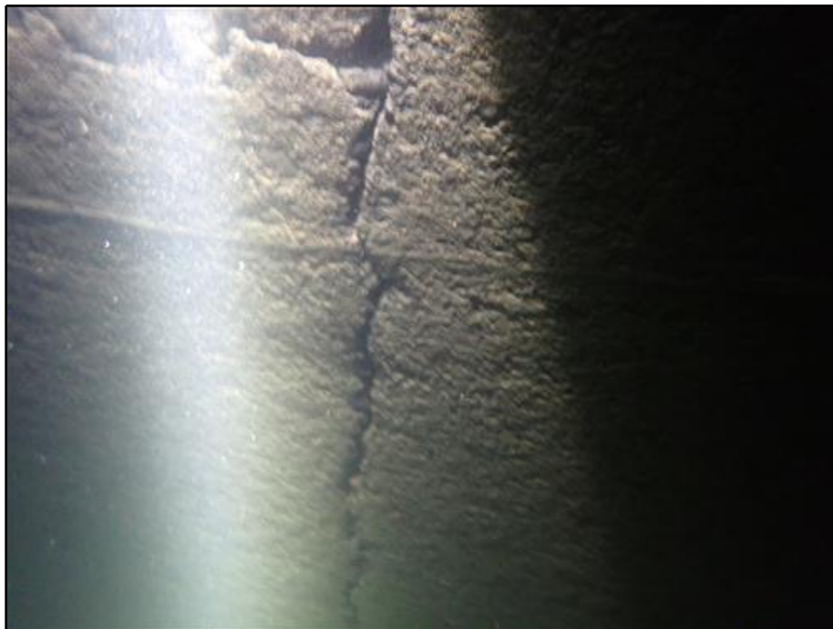
14. South Footing, 18'-0" from East End - Crack, Full Height x 1/4" Wide
