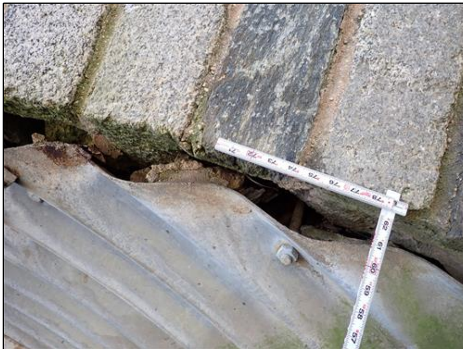
12. West Spandrel Wall/Arch Plate Interface - Missing Mortar
