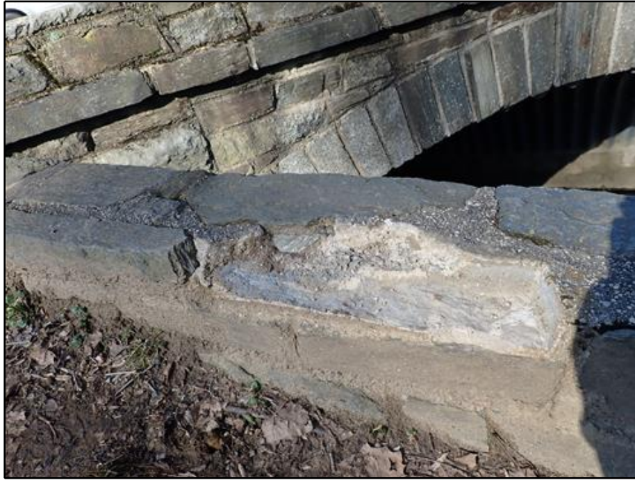
13. Southeast Wingwall - Missing Stone on Top Face Approximately 5'-0" from Spandrel Wall
