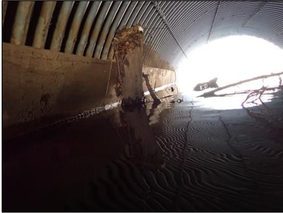
19. Channel - Debris Buildup at Interface Between South Footing and Utility Pipe
