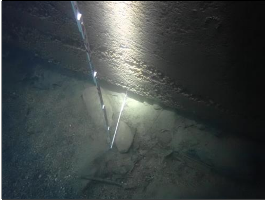
17. South Footing - Typical Undermining
