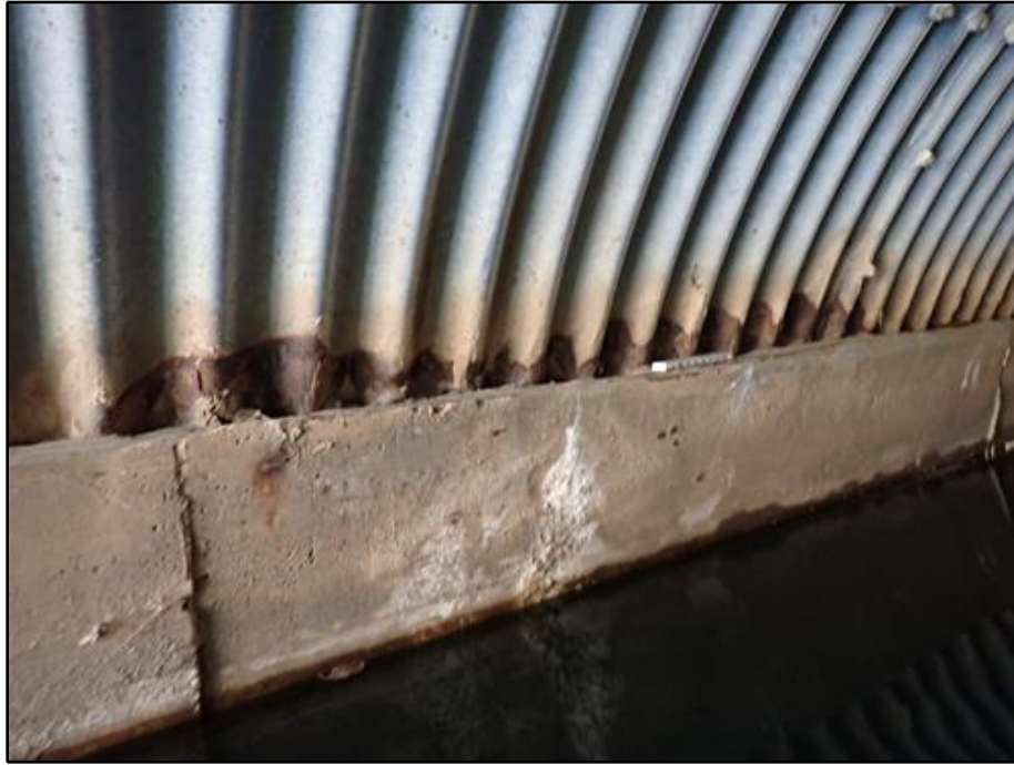
11. Arch - Corrosion along Base Above North Footing at West End
