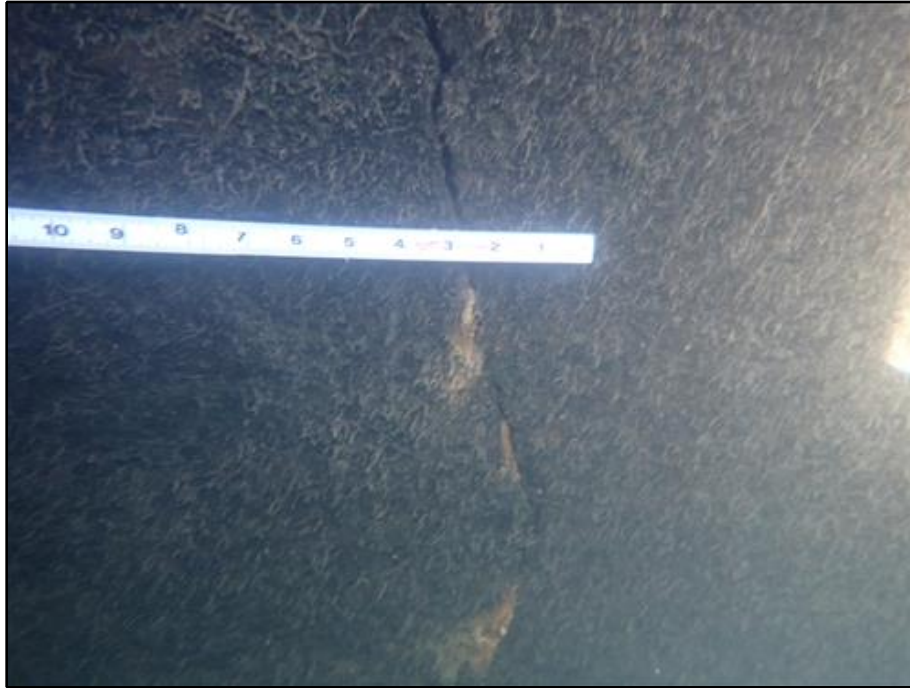
15. North Footing, 7'-0" from East End - Crack, Full Height x 1/8" Wide
