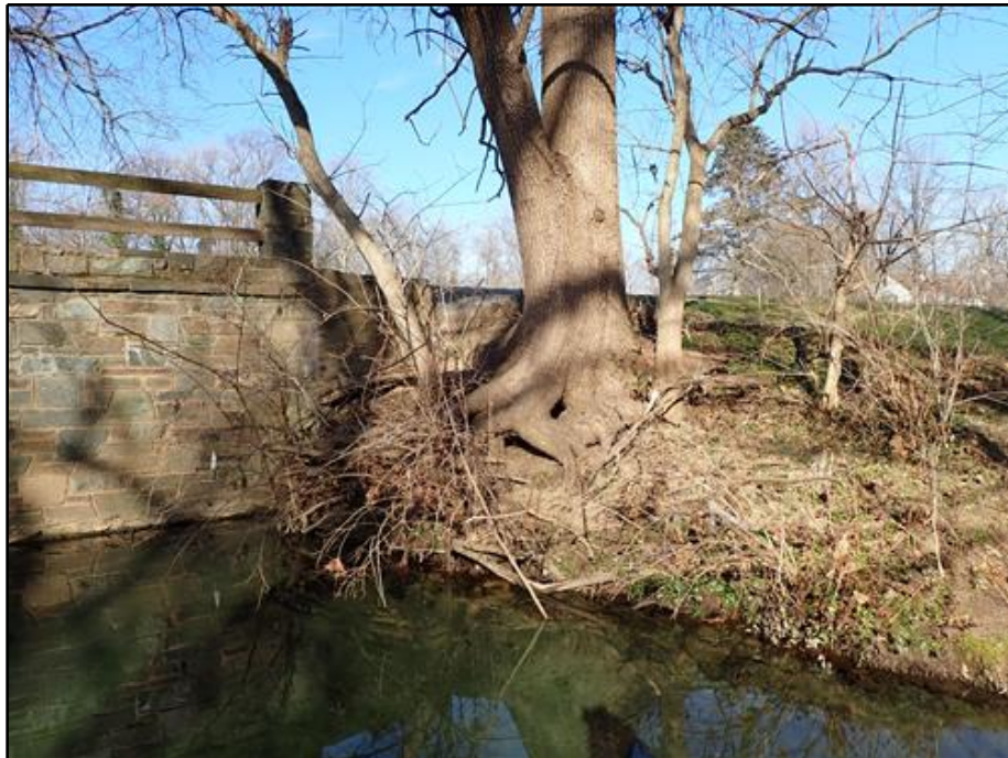
18. Northeast Embankment - Exposed Tree Roots
