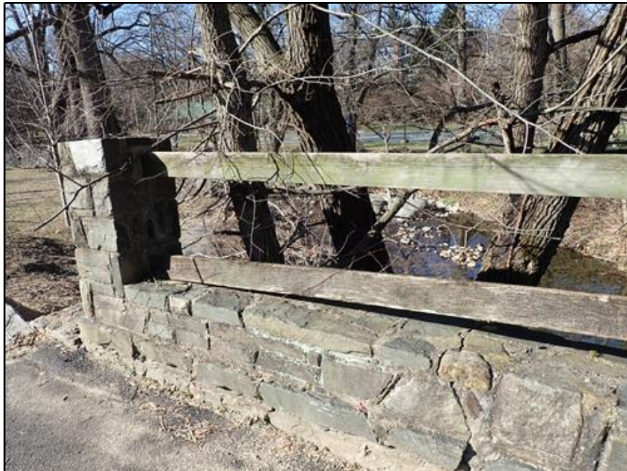
10. West Railing - Lower Timber Detached Between Pilasters 4 and 5
